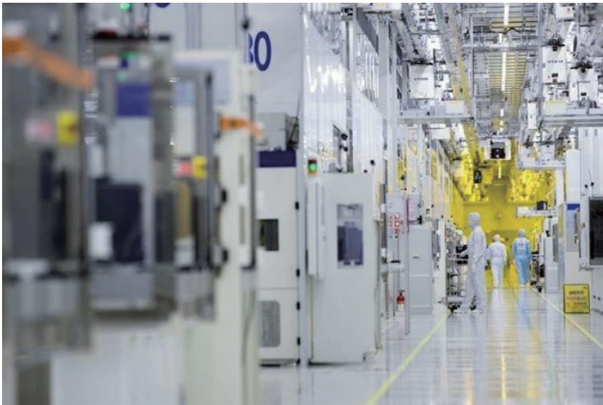
Figure 2 Semi-conductor plant in Korea
